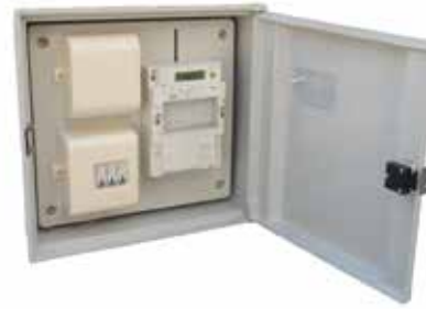
House Meter with SMC BOX
